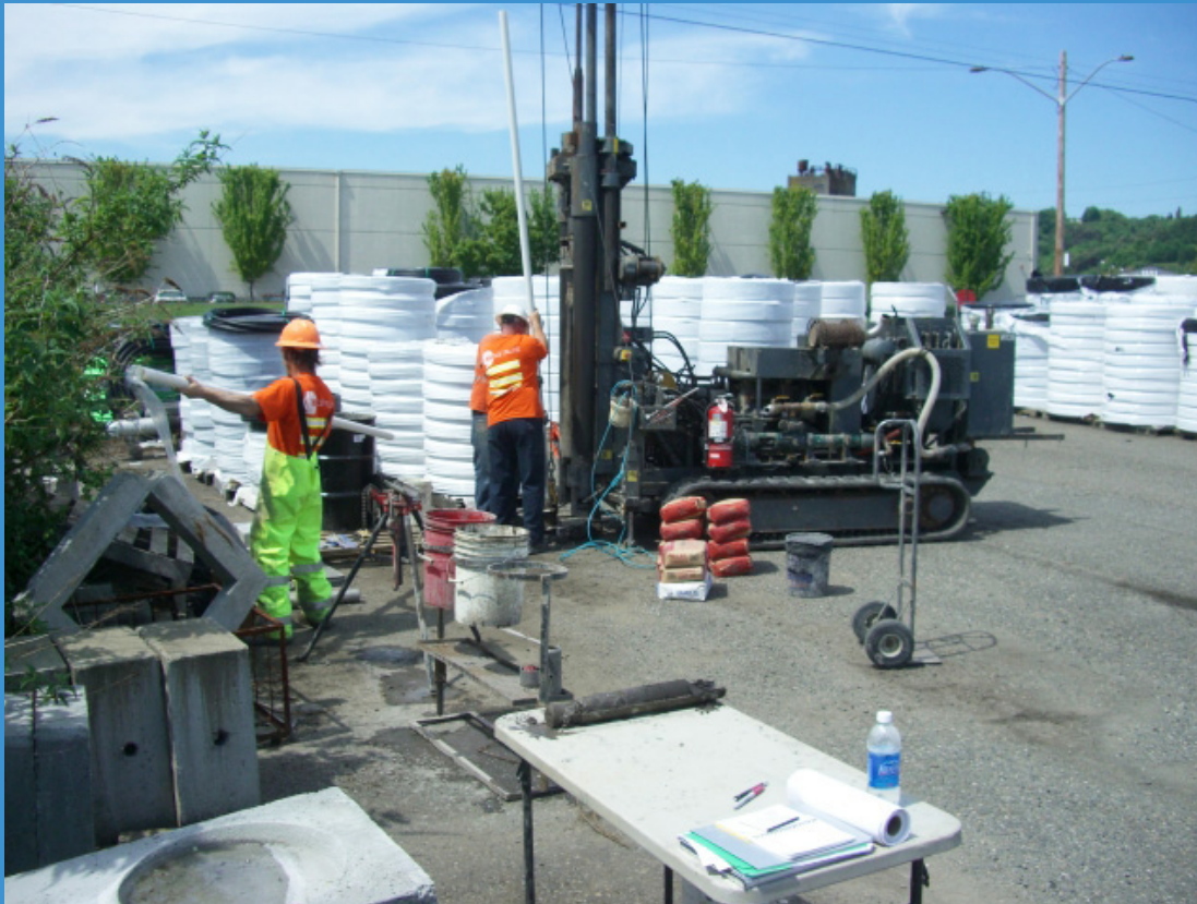
Hydrogeologists Logging Station
